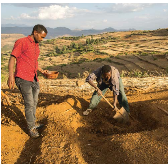
A farmer (Emwodeh Geze) is constructing his own ring-basin infiltration pit and perma-garden in his backyard with support by one of the trainers (Mengist Dereje) in Gakiew village, Wag-Himera Zone (2017)
