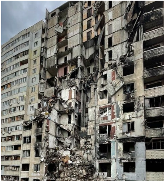
Damaged Khrushchevka building in Kharkiv (D. Wyss)
