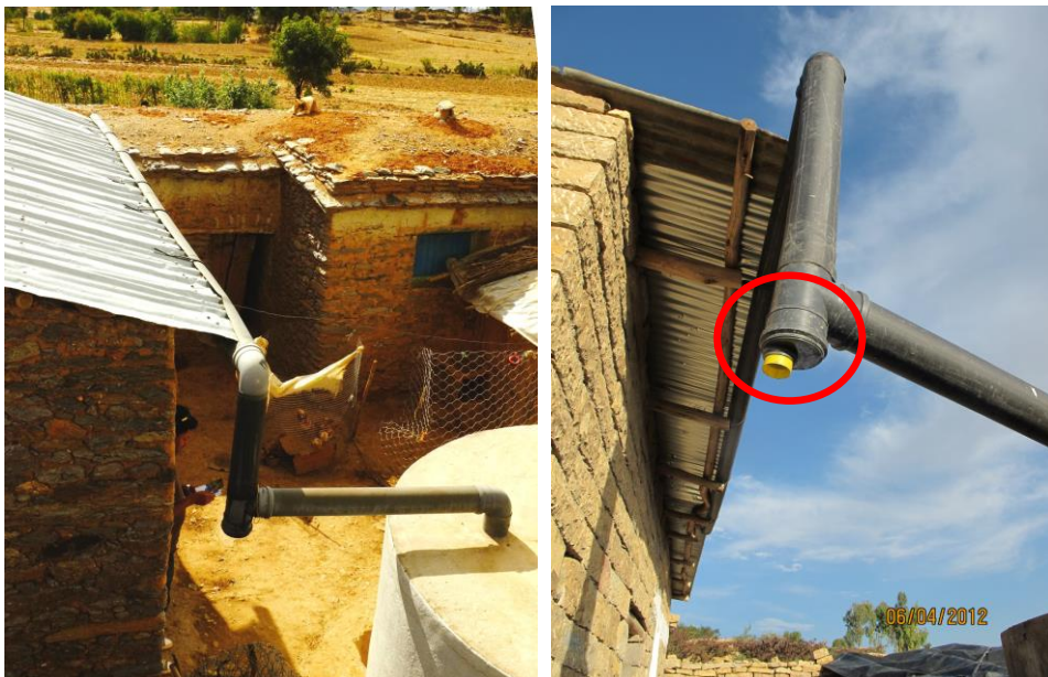
Pictures above: Roof catchment and first splash discharge installation
